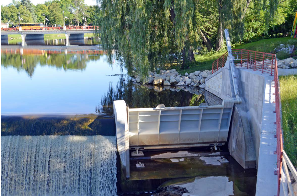
Figure 1. Hydraulically operated crest gate on the Milwaukee River in Grafton, WI (Photo: Ayres)
