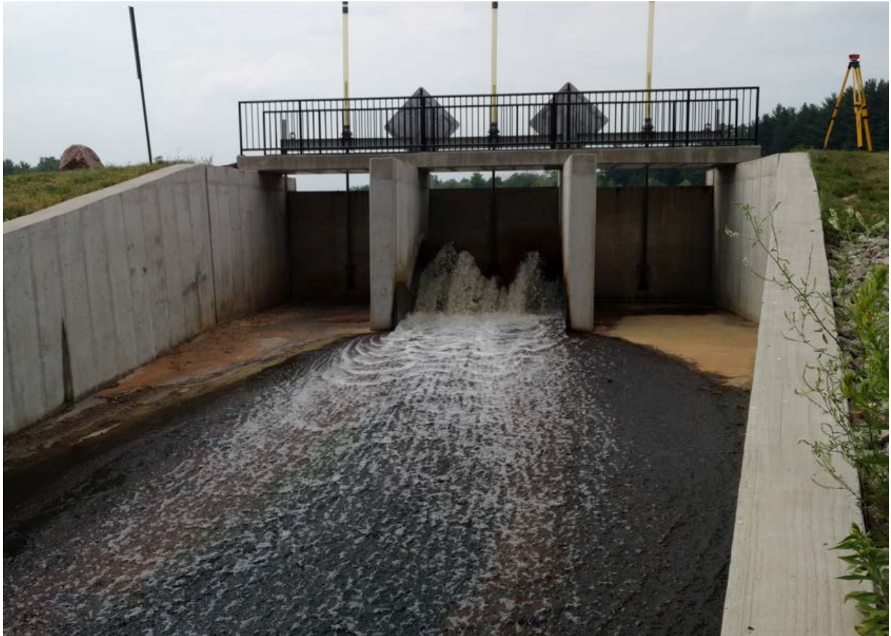
Figure 3: Three stainless steel slide gates in Ogdensburg, WI (Photo: Ayres)
